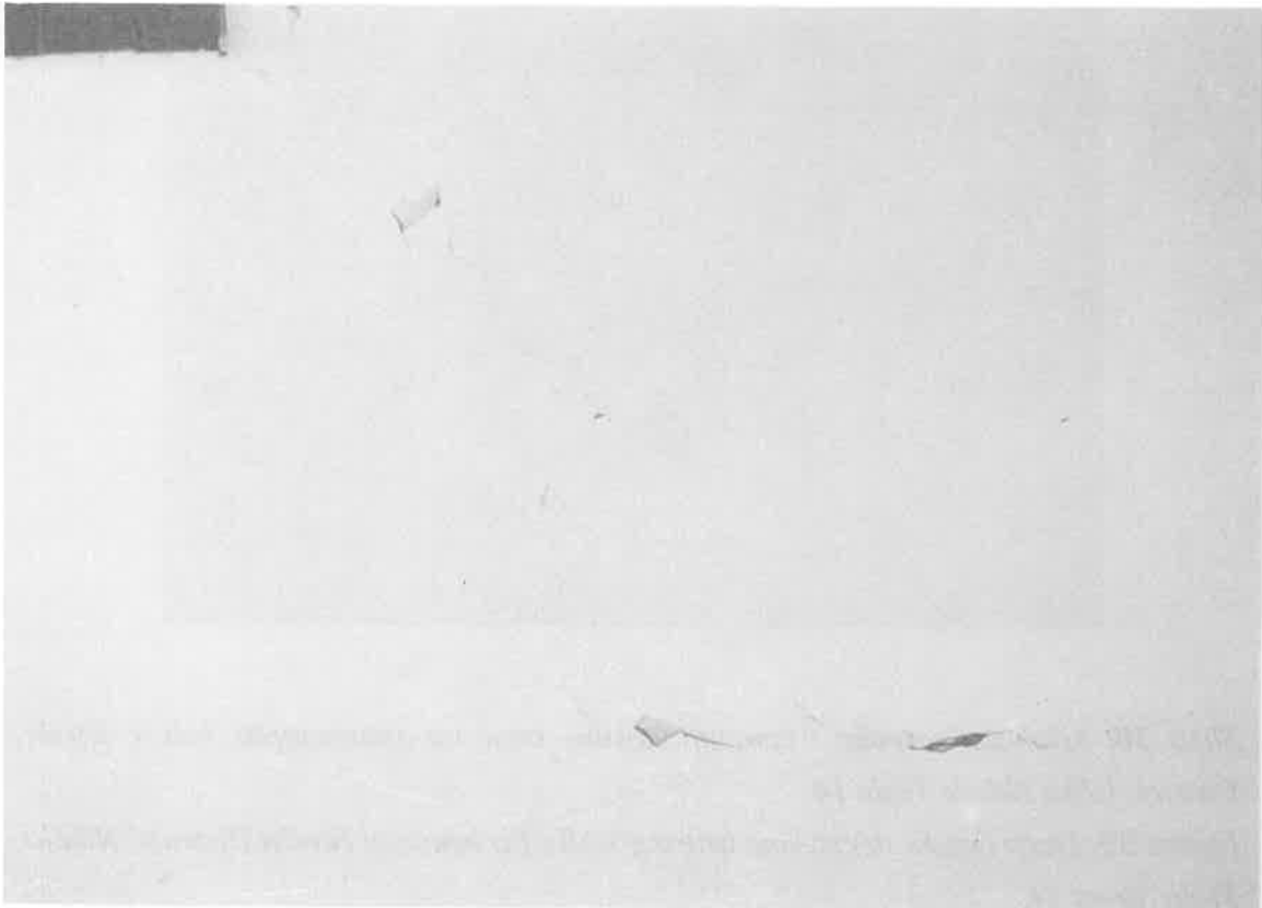
Slika 29: Razpoke in odpadanje koščkov ometa v stanovanjski hiši v Ilirski Bistrici, Ulica Nikole Tesle 14. Figure 29: Cracks and fall of small pieces of plaster in a building in Ilirska Bistrica, Nikola Tesla Street 14.
