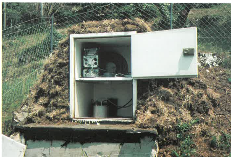
Slika 3. V omarici, ki je postavljena na skalnati podlagi, je bil v prvi polovici leta postavljen prenosni seizmograf Reftek 72A-07/DAT s senzorjem Guralp CMG-40T (foto: R. Vidrih). Figure 3. In a metal case set up on the rock base, a Reftek 72A-07/DAT portable seismograph with a Guralp CMG-40T sensor was installed during the first half of the year (photo: R. Vidrih).
