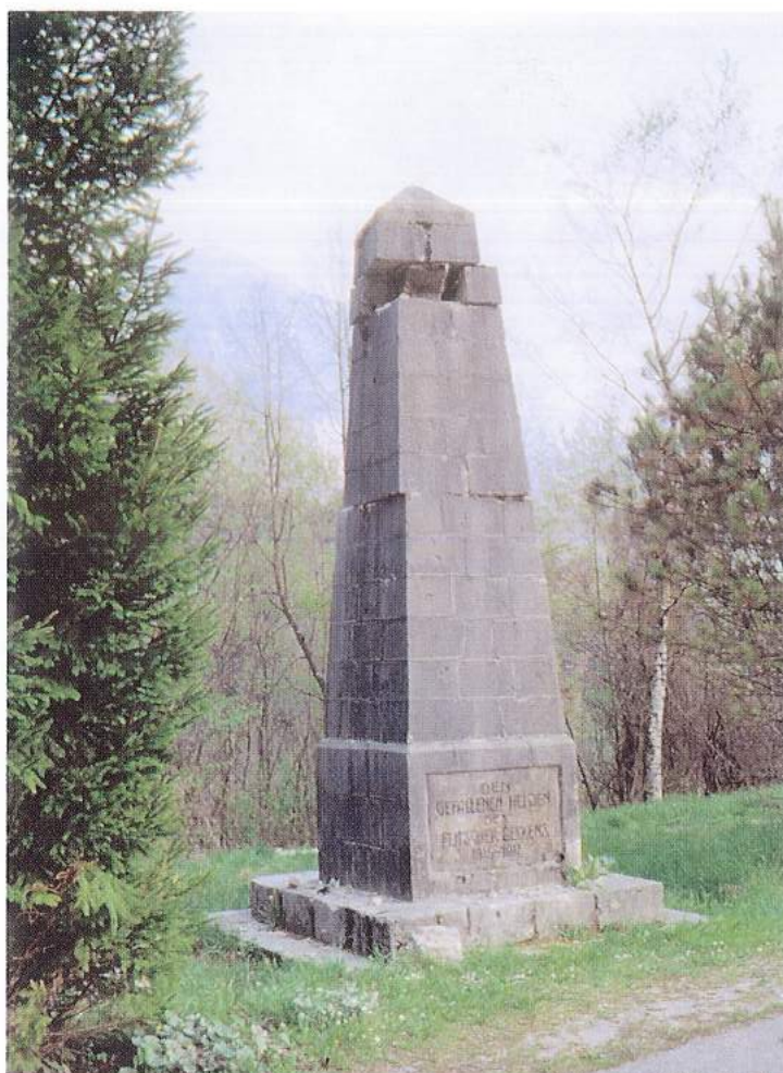
Slika 8. Zasuk kamnitih blokov na spomeniku pred Bovcem (poškodbe 3. do 4. stopnje) Figure 8. Twisted stone blocks on the monument outside Bovec (damage of grades 3 and 4).
