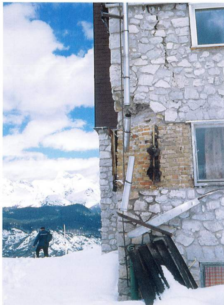
Slika 7. Poškodbe Ski hotela na Voglu (poškodba 3. stopnje) Figure 7. Damage to Ski hotel on Mount Vogel (damage of grade 3).
