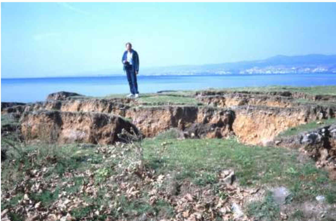
Slika 23. Razpoke v preperini in posedki ob morski obali (spodaj) (foto: R. Vidrih). Figure 23. Cracks in the weathering cover and subsided areas at the seacoast (below) (photo: R. Vidrih).
