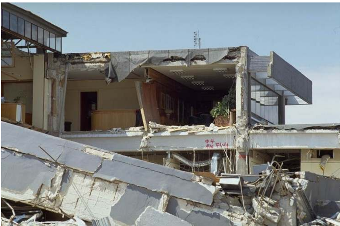
Slika 6. Detajl porušene tovarne. Figure 6. Detail of the collapsed factory.
