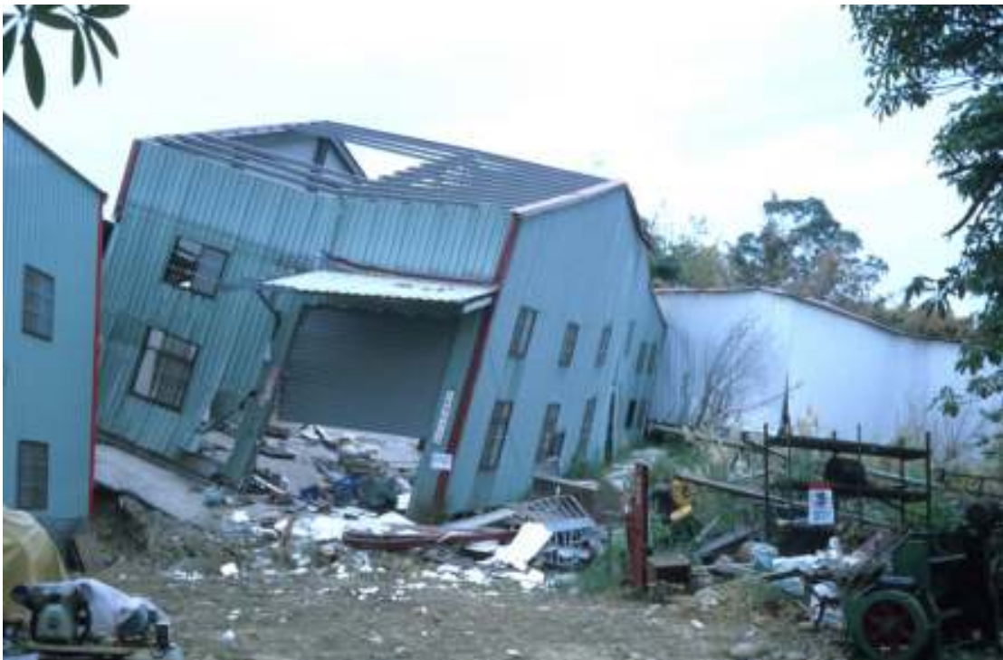
Slika 7. Stanovanjska hiša na prelomu ne more vzdržati obremenitev, pa tudi deformacije tal ne (vertikalni premiki so bili tudi do 8 m) (spodaj) (foto: R. Vidrih). Figure 7. The residential house at the fault cannot bear the burden, nor the deformation of the ground (there were vertical offsets of up to 8 m) (below) (photo: R. Vidrih).
