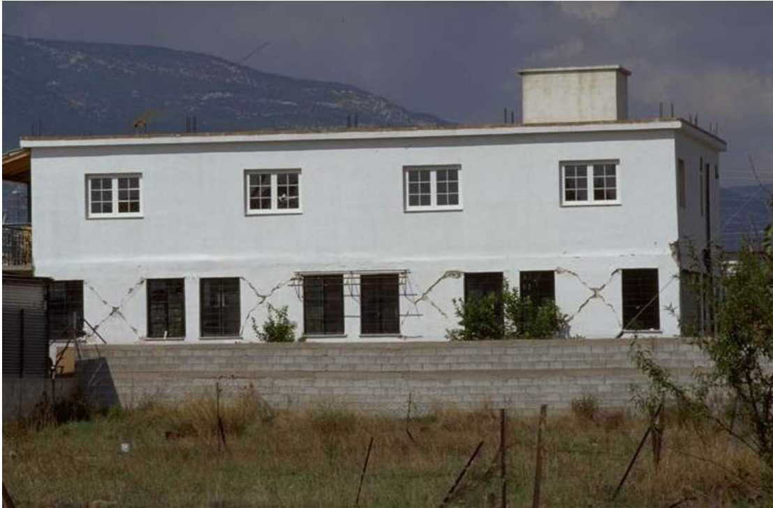
Slika 7. Mnoge poškodbe objektov vzdolž ulice Dekelias v Atenah. Figure 7. Several damaged buildings along Dekelias road (Athens).
