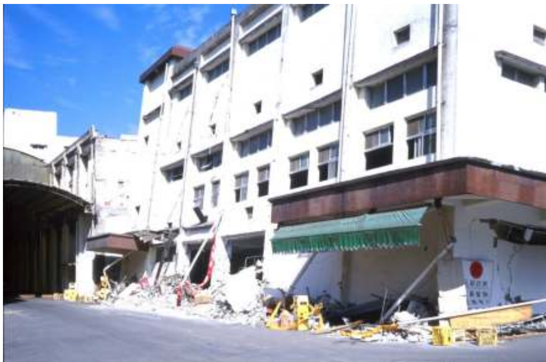
Slika 5. Vzrok porušitve industrijskega objekta je bila mehka etaža (foto: R. Vidrih). Figure 5. The reason for the collapse of the industrial building was soft storey (photo: R. Vidrih).
