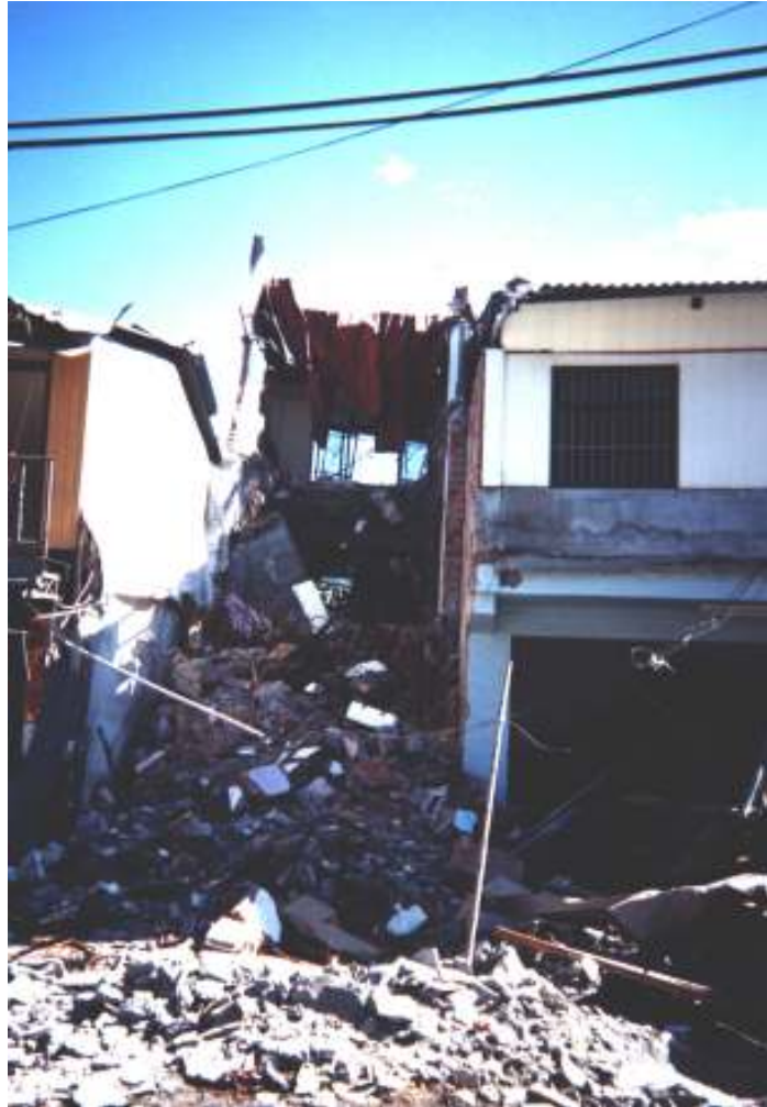
Slika 15. Popolnoma porušena stanovanjska zgradba (foto: M. Godec). Figure 15. Completely destroyed residential building (photo: M. Godec).
