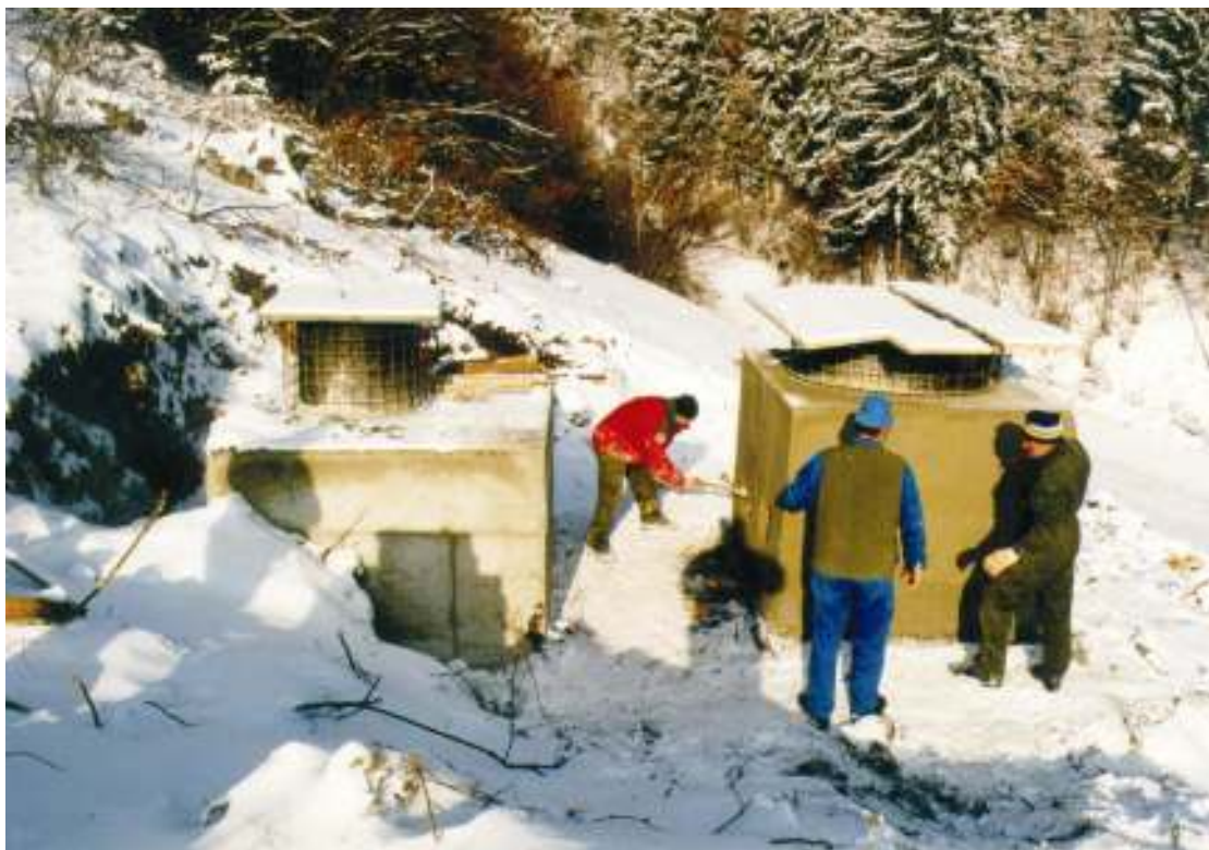
Slika 10. Stanje del na lokaciji Goliše ob prekinitvi del 14. decembra 2001 (opravljena betonska dela, onemogočeno polaganje elektroenergetskega kabla zaradi nizkih temperatur). Figure 10. Goliše station on 14 December 2001, when works had to be stopped (concreting works completed, laying of the electro-energetic cable was impossible due to low temperatures).
