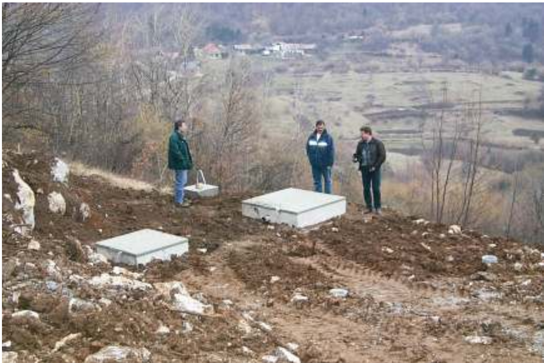
Slika 16. Okolico obeh jaškov je potrebno še zatraviti in ograditi. Figure 16. The shafts' surrounding area needs to be grassed and fenced.
