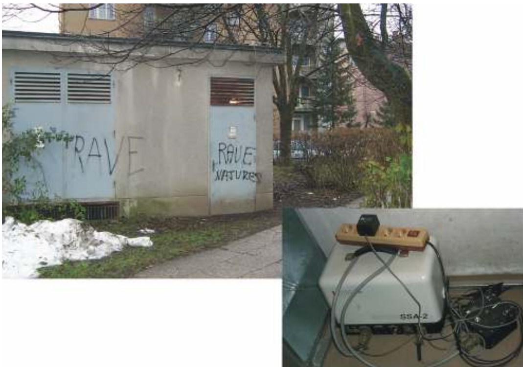
Slika 9. V transformatorski postaji pri FGG je nameščen akceleroграф SSA-2. Figure 9. Accelerograph SSA-2 is set up in the building near the Faculty of Civil and Geodetic Engineering in Ljubljana.
