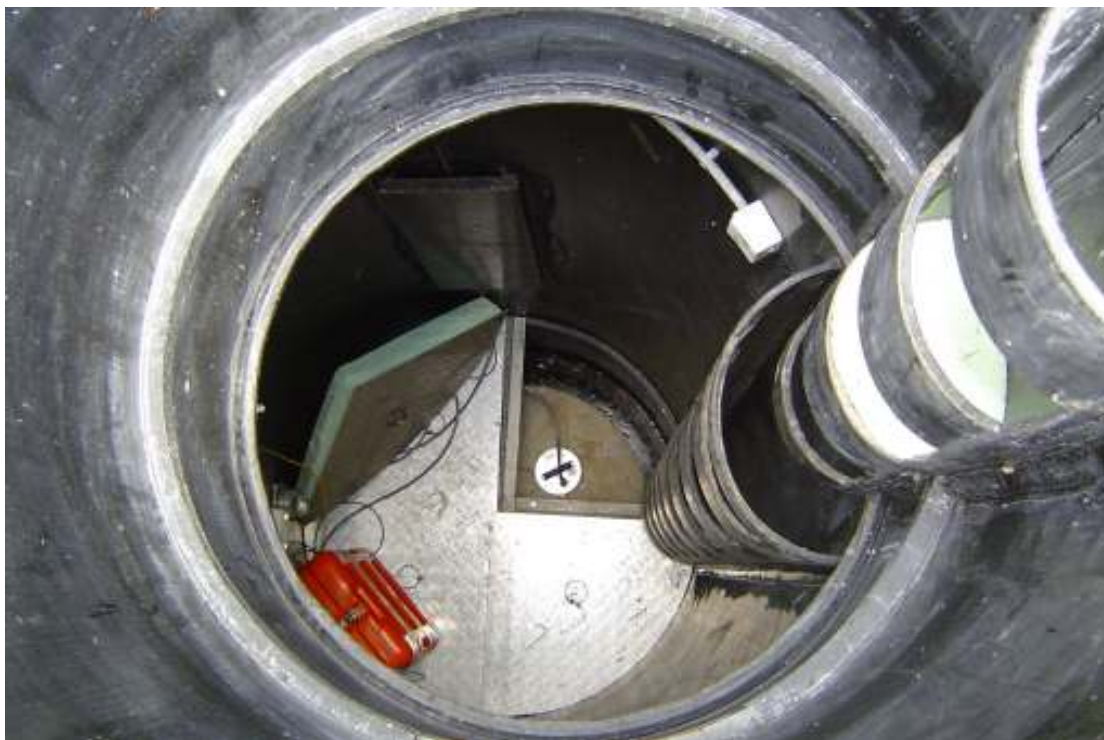
Slika 3. Seizmični jašek s seizmometrom in zajemalno enoto Figure 3. Seismometer and acquisition unit are set up in seismic shaft
