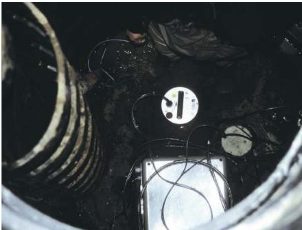
Slika 6. Referenčni senzor je postavljen na dno jaška Figure 6. The reference sensor is set up on the bottom of the well
