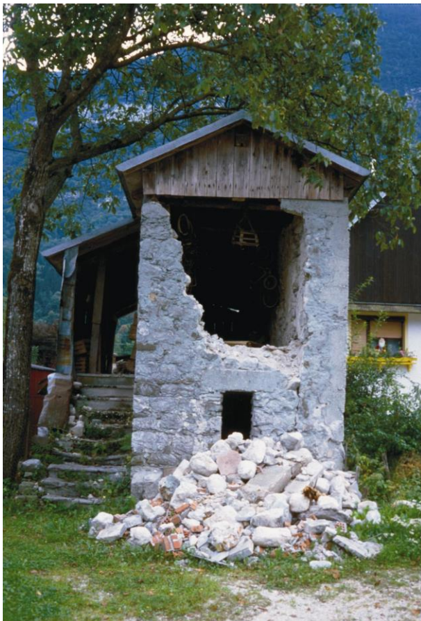
Slika 22. Močno poškodovan objekt v vasi Čezsoča. Figure 22. Destroyed building in the village of Čezsoča.
