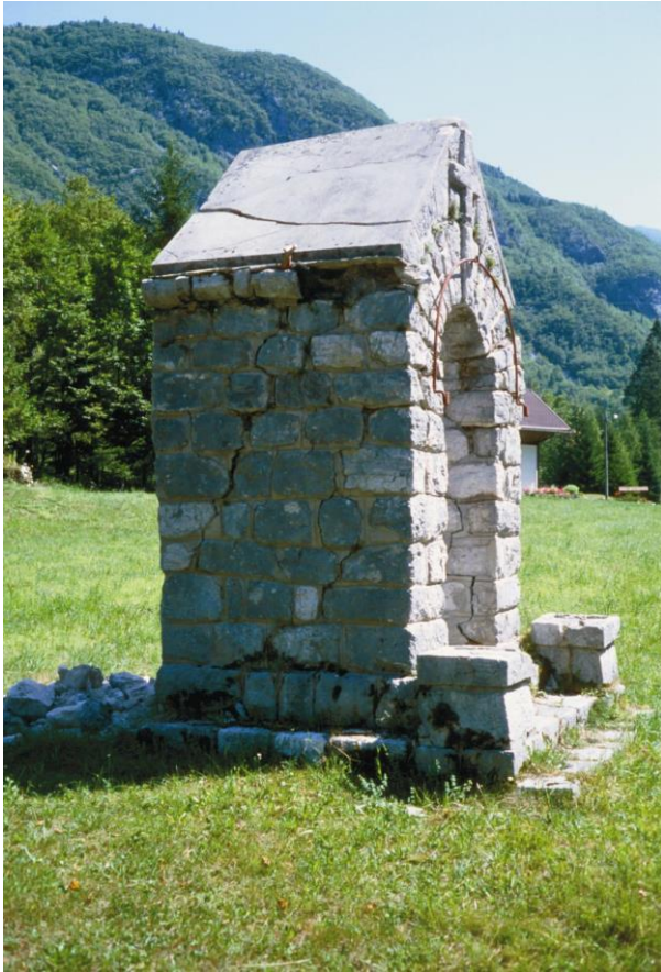
Slika 21. Močno poškodovana kapelica v vasi Soča. Figure 21. Severely damaged chapel in the village of Soča.
