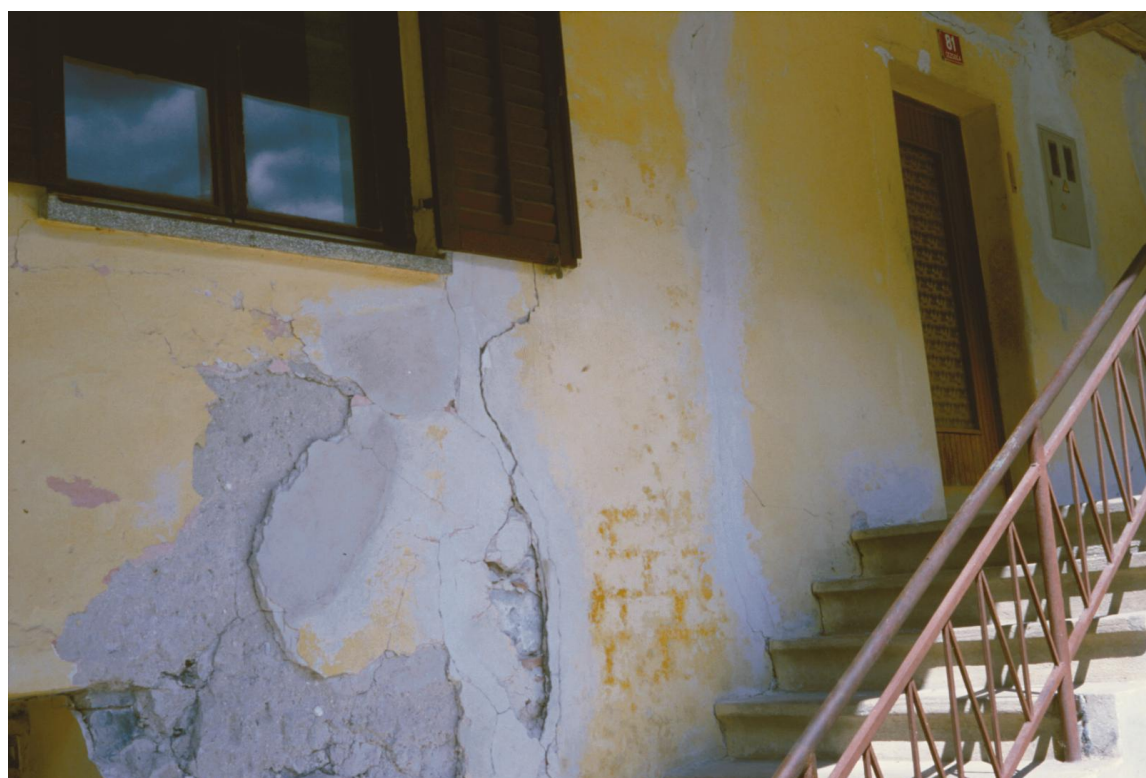
Slika 14. V vasi Čezsoča je bilo poškodovanih veliko starejših objektov. Figure 14. A large number of older buildings were damaged in the village of Čezsoča.
