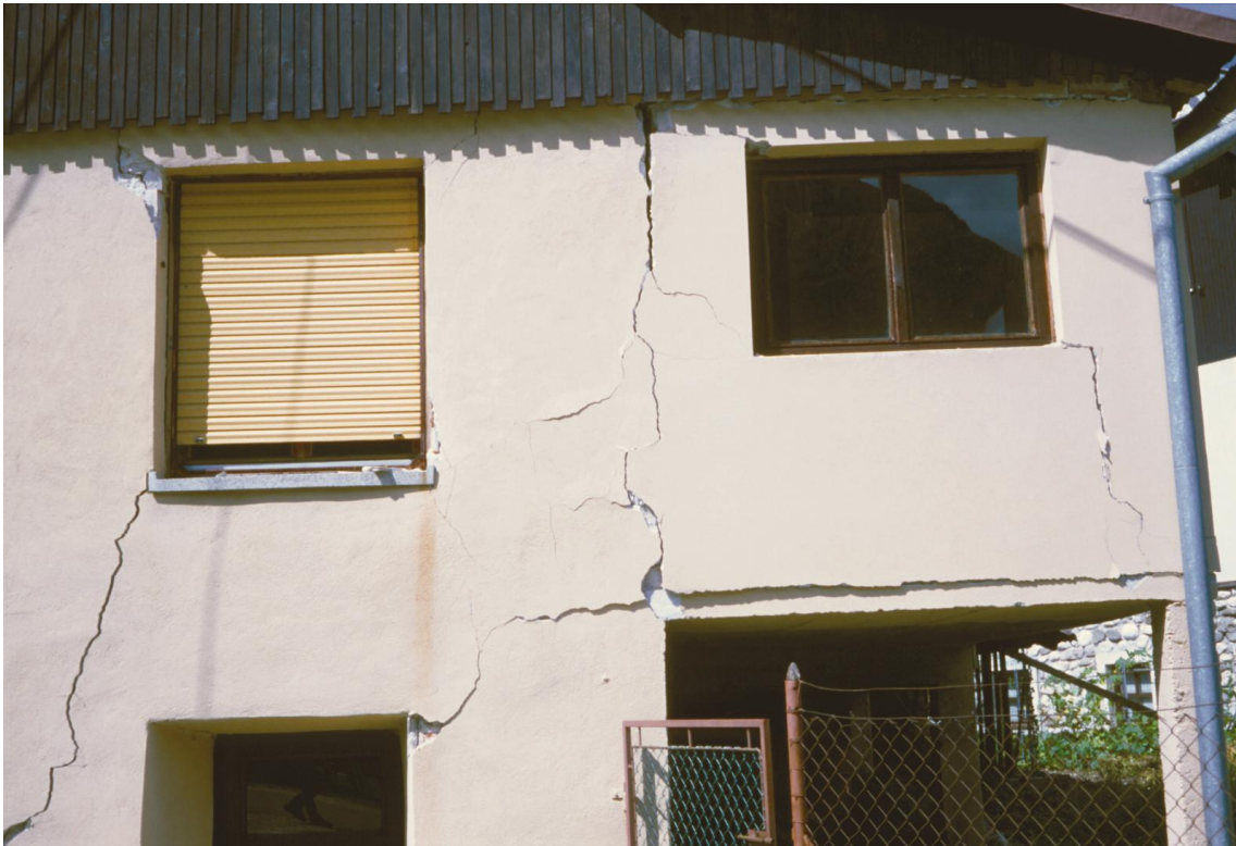
Slika 15. Močno poškodovana hiša v Čezsoči kaže na neprimerno dozidavo prizidka. Figure 15. Severely damaged house in Čezsoča indicates inadequate construction of the annex.
