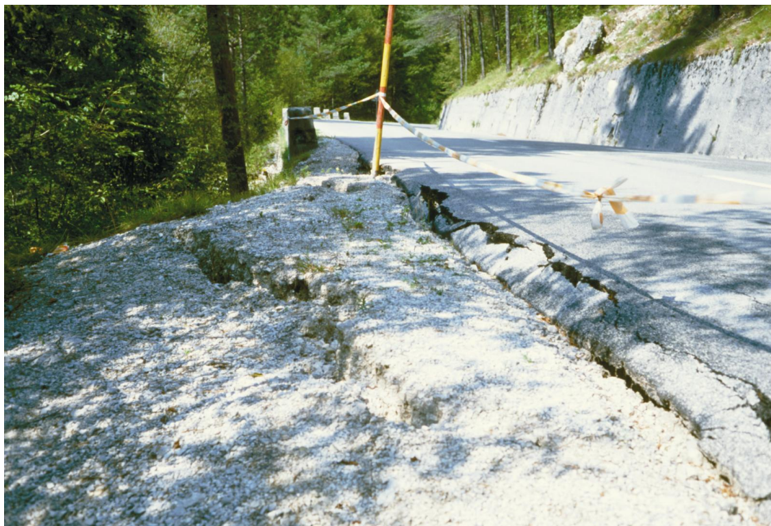
Slika 23. Posedek ob strmem bregu na robu ceste v bližini Golobarske žičnice. Figure 23. Subsiding of the ground at the roadside near the Golobar cableway.
