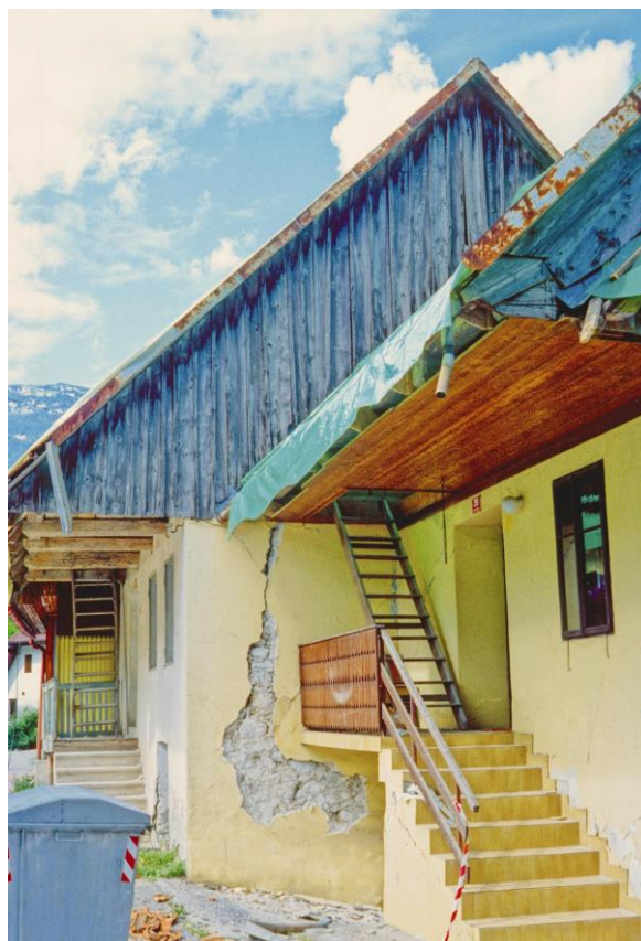
Slika 18. Zaradi slabih seizmogeoloških razmer so bili učinki potresa v nekaterih predelih za celo stopnjo višji. Nekateri objekte v Čezsoči je bilo treba podreti. Figure 18. Because of poor seismological conditions, the effects of the earthquake were one whole level higher. It was necessary to demolish some buildings in Čezsoča.
