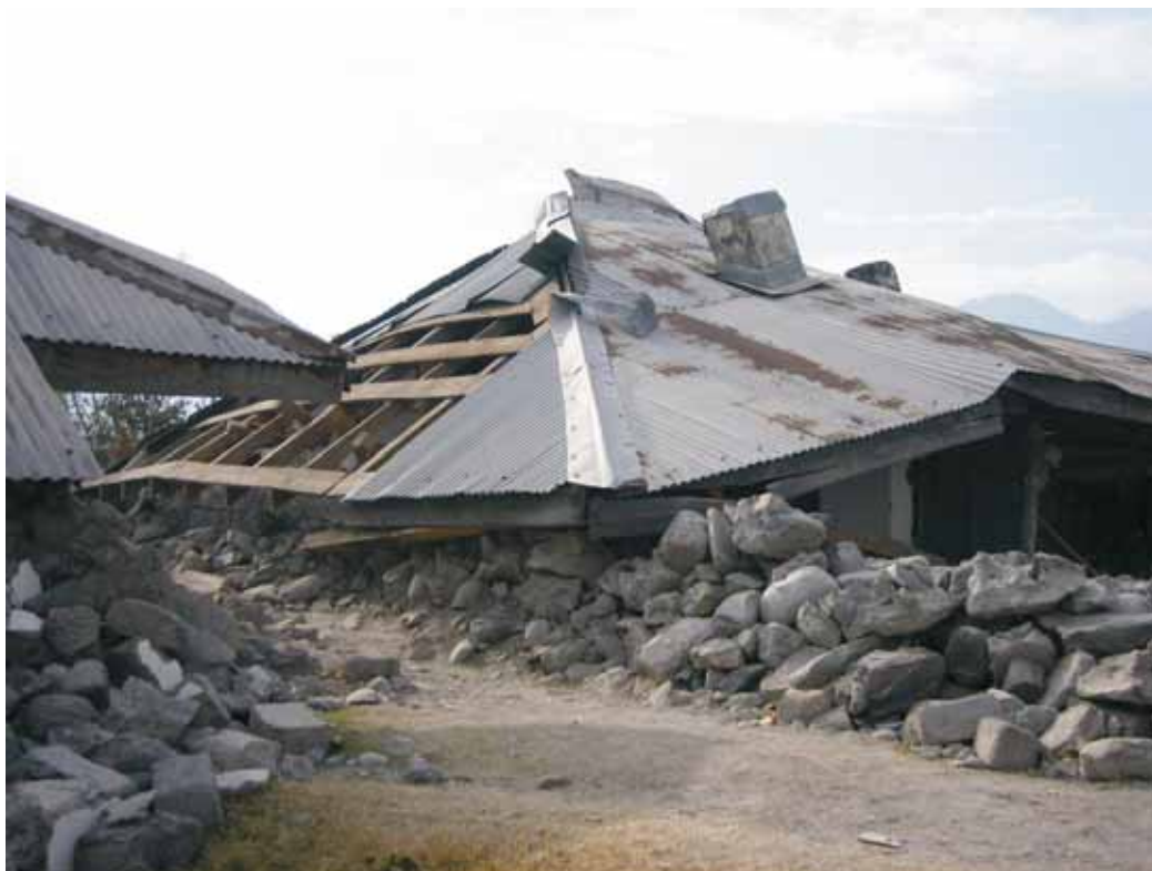
Slika 20. Na poti v Muzaffarabad: porušena šola. Figure 20. On the way to Muzaffarabad: collapsed school building.
