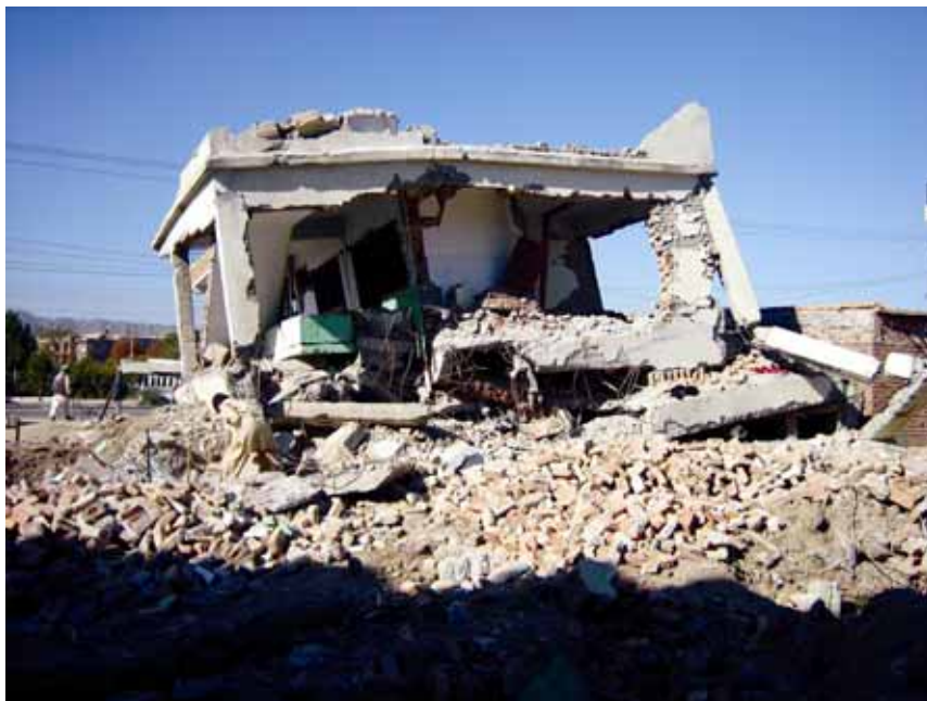
Slika 11. Abbotabad: ostanki armiranobetonske stavbe z zidanimi opečnimi polnili. Figure 11. Abbotabad: debris left of an r.c. frame structure with masonry infill walls.
