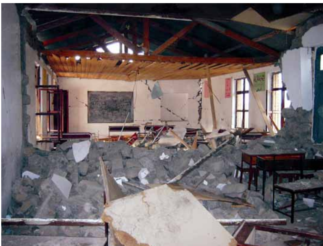
Slika 21. Na poti v Muzaffarabad: lesena strešna konstrukcija šole, porušeni prečni zid in močno poškodovano obodno zidovje. Figure 21. On the way to Muzaffarabad: wooden roof structure of a school building, collapsed cross wall and heavily damaged peripheral walls.
