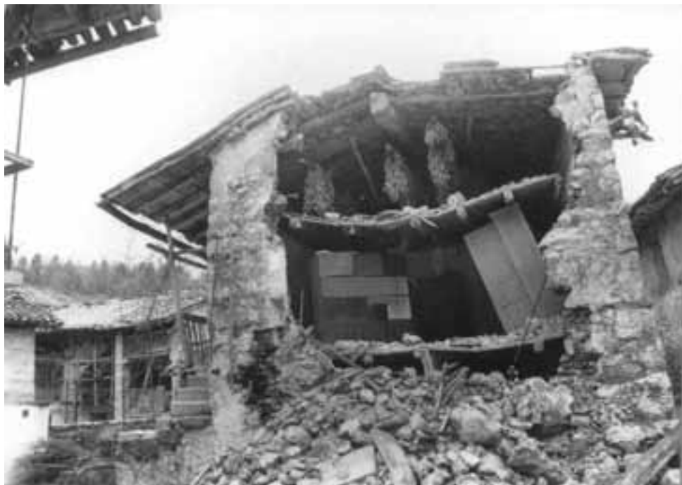
Slika 1. Poškodovan objekt v Breginju (Arhiv ARSO, Urad za seizmologijo in geologijo). Figure 1. Damaged building in Breginj (Archive ARSO, Seismology and Geology Office).
