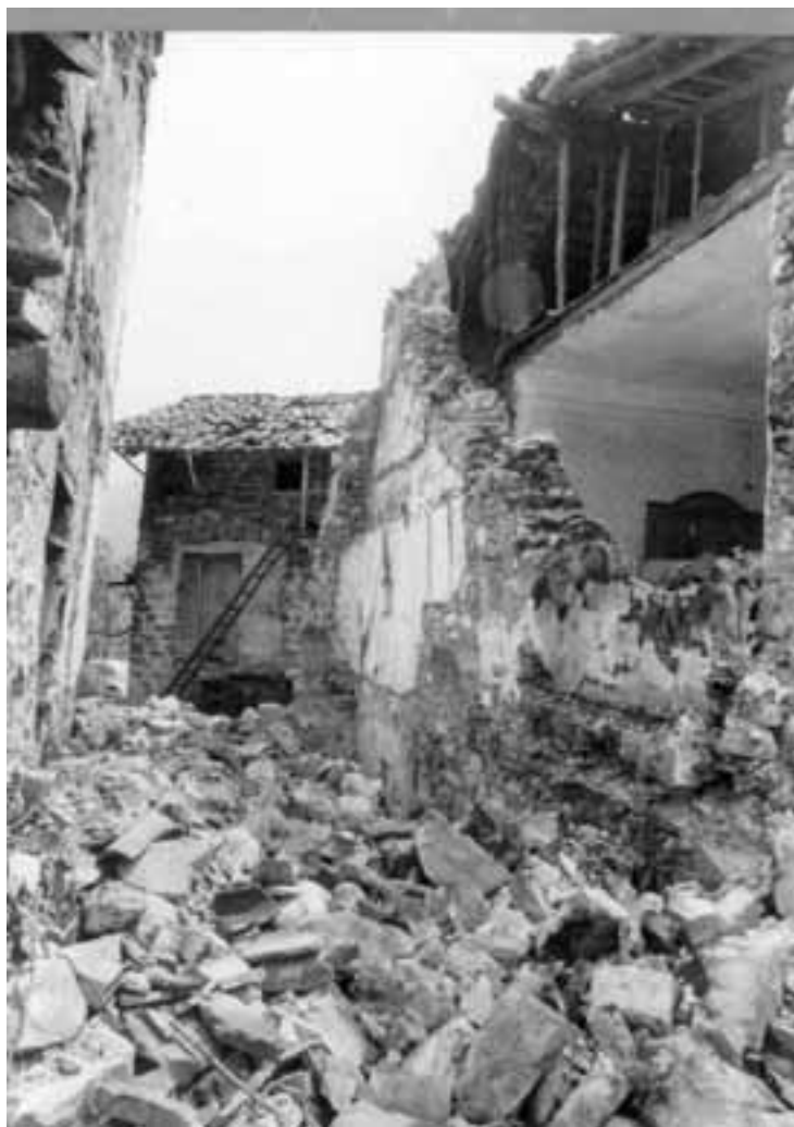
Slika 3. Porušeni objekti v Breginju (Arhiv ARSO, Urada za seizmologijo in geologijo). Figure 3. Demolished buildings in Breginj (Archive ARSO, Seismology and Geology Office).
