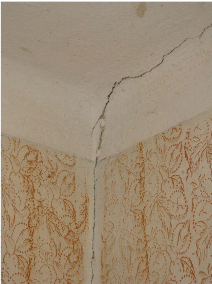
Figure 6: Fall of small pieces of plasters (photo: M. Godec)
