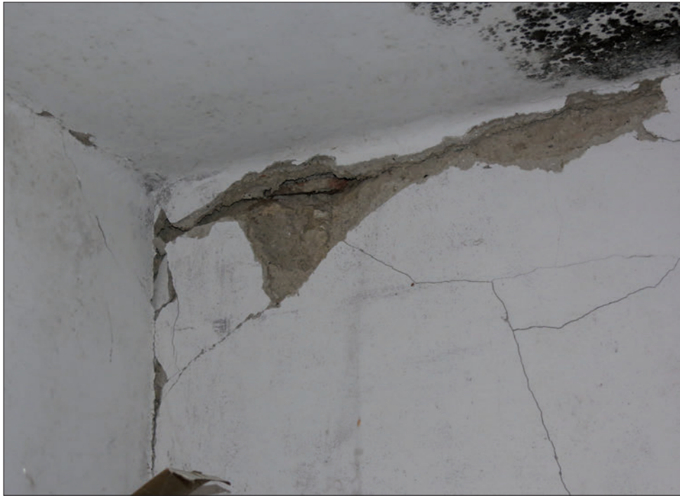
Slika 10: Široke in globoke razpoke nosilnega zidu na Vinjem Vrhu (foto M. Godec) Figure 10: Large and extensive cracks in bearing wall at Vinji Vrh (photo M. Godec)
