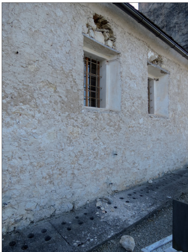
Figure 13: Deep crack in the outer wall of the church at Bušeča vas (photo M. Godec)
