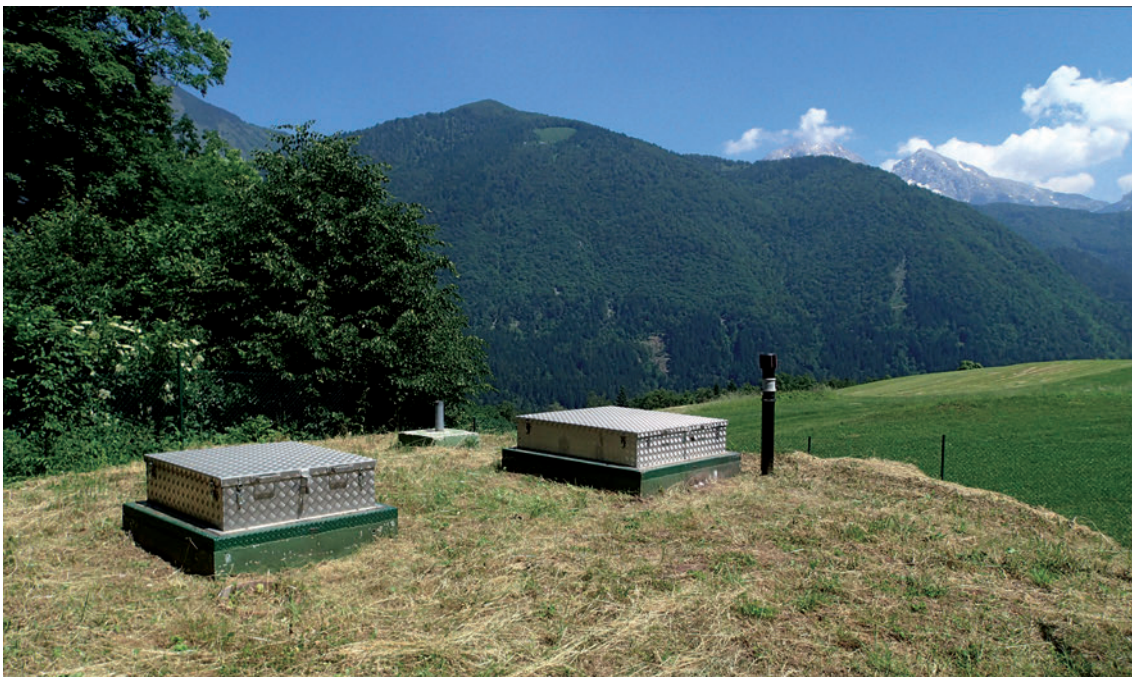
Slika 3: Pogled na potresno opazovalnico MOZS, kjer smo zamenjali komunikacijsko in seizmološko opremo ter namestili sistem za samodejno črpanje vode (foto: I. Tasič) Figure 3: View of seismic station MOZS where the new communication and acquisition equipment, along with automatic water pumping system was installed. (Photo: I. Tasič)
