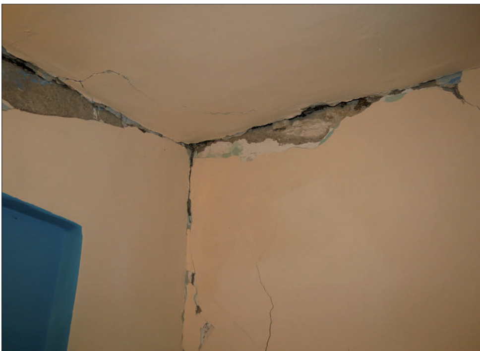
Slika 6: Široke in globoke razpoke na stikih nosilnih zidov in stropa na Stojanskem Vrh (foto M. Godec) Figure 6: Large and extensive cracks in the joints of walls and ceiling at Stojanski Vrh (photo M. Godec)
