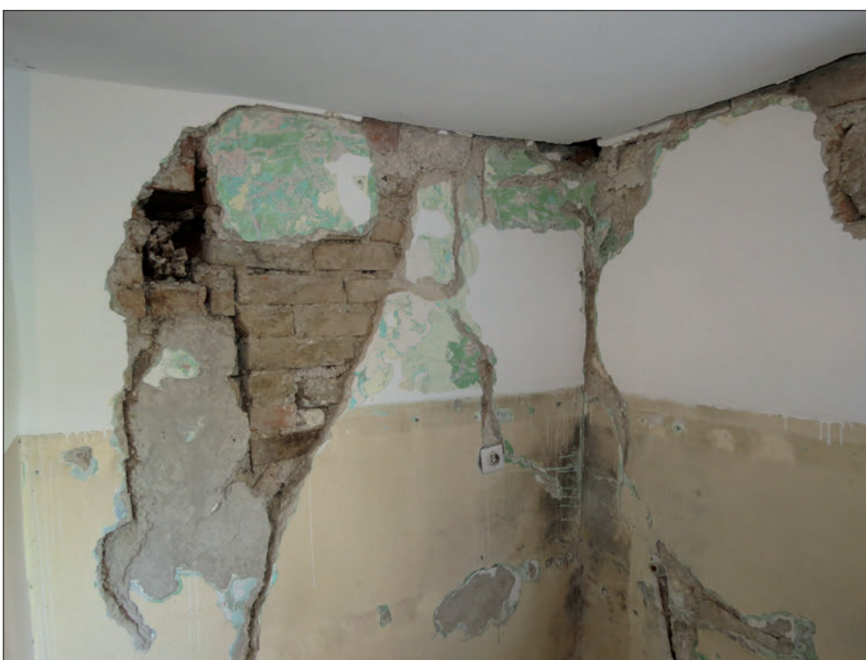
Slika 7: Široke in globoke razpoke nosilnih zidov na Stojanskem Vrh (foto M. Godec) Figure 7: Large and extensive cracks in bearing walls at Stojanski Vrh (photo M. Godec)
