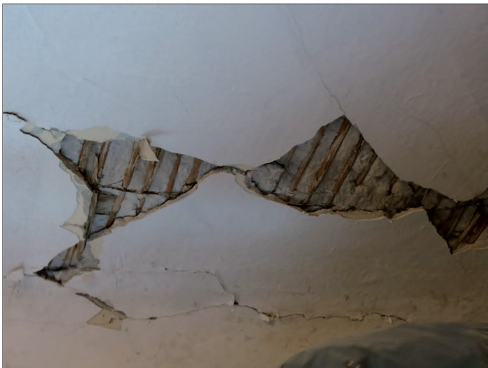
Slika 11: Odpadli večji kosi ometa na stropu v Vinjem Vrhu (foto M. Godec). Figure 11: Large pieces of plaster falling off the ceiling in Vinji Vrh (Photo M. Godec).
