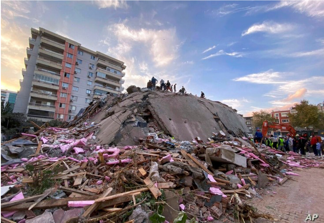
Slika 6. Popolnoma porušena zgradba v Izmirju, Turčija, ob potresu 30. oktobra 2020. (vir: https://www.voanews.com/europe/powerful-quake-strikes-major-turkish-city-greek-islands ) Figure 6. Building that collapsed during the 30 October 2020 earthquake in Izmir, Turkey (Source: https://www.voanews.com/europe/powerful-quake-strikes-major-turkish-city-greek-islands )
